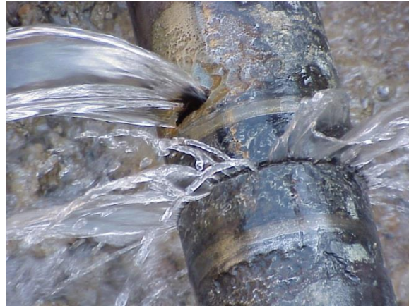
Photo: Broken Water Main
