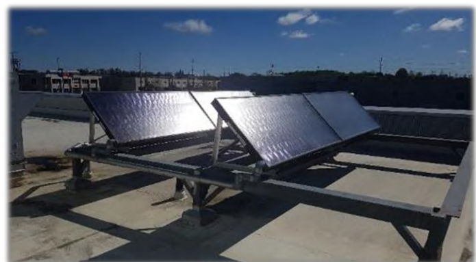
Solar Thermal System
