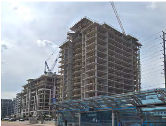
380-398 HIGHWAY 7, RICHMOND HILL Eight Storey Residential Building Population 1 : 660 Jobs 2 : 25 Gross Area 3 : 2.4 ha
